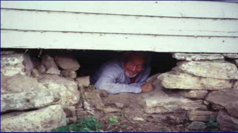
Professor Woodcock investigates the foundation under the western portion of the original structure.
