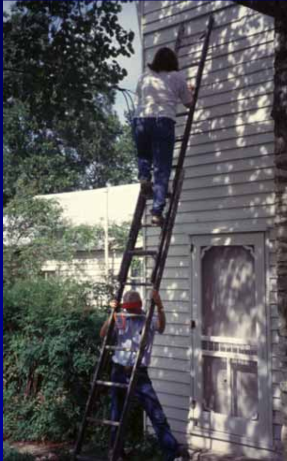
Laura Brown climbs the ladder to get additional measurements of the eaves, while Larry Reiter braces the ladder.
